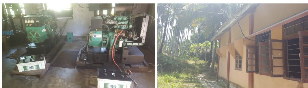
Figure 2.6: Diesel generators and generator house on Rutland
